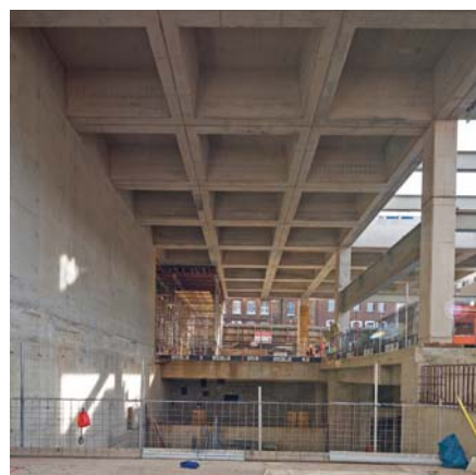
ABOVE: Exposed concrete surface finish with two-way spanning ribs (Crossrail Farringdon Station).
