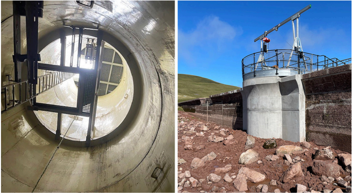
(left) Lined tower – Courtesy of HR Wallingford, and (right) Completed external lining – Courtesy of Morgan Sindall
