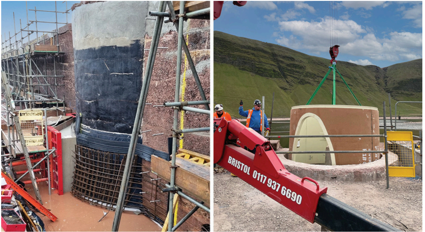
(left) External lining construction – Courtesy of Arup, and (right) Installation of GRP lining from iLine Technologies Ltd – Courtesy of Morgan Sindall
